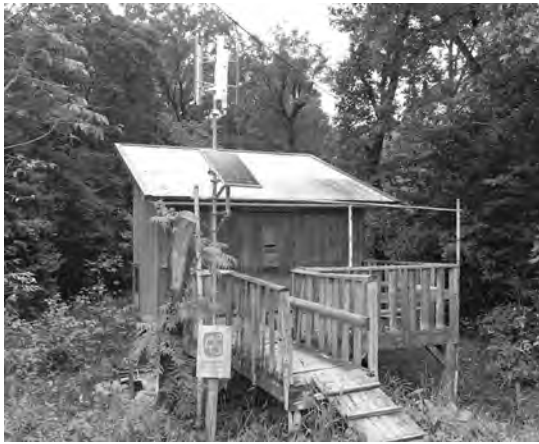
Figure 17. Solar panels and windpower generator (2016)
