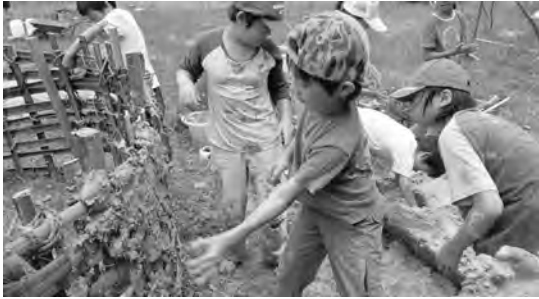
Figure 11. Children using the flatland soil to build a house in the outdoor experience workshop “Forest” (2009)
